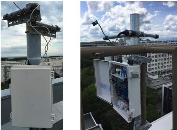
Fig. 13. Example of Blitzortung installation (Left: Fujisawa city, Right: Sendai city)
